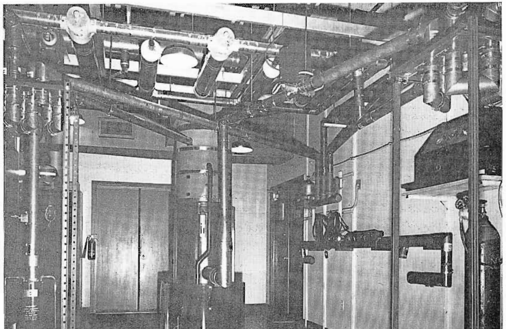
Fig. 30. The motor driven coaxial switches mounted on rear wall are to switch the TT-25CL (or the TT-6AL Auxiliary) to the antenna. The manually operated coax switches are used to interchange the two TT-6AL's as drivers and to connect the transmitters to the dummy loads.
