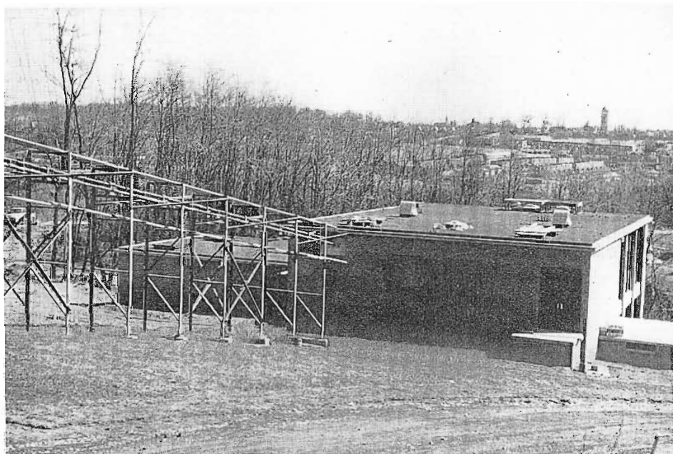
FIG. 13. The transmission line of each station is run to the tower on a steel frame as shown here at the WBAL building. Small pipes have been mounted over the lines to prevent damage from falling ice.
